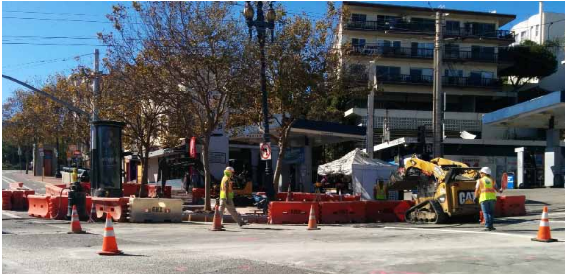
The city has been aggressively pursuing its mandate to repair and change San Francisco's roadways and related pedestrian amenities. PHOTOS: JOHN ZIPPERER
